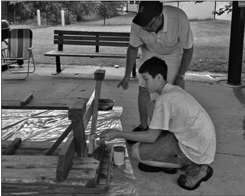
Above: TASC volunteers paint a picnic table in the Adams Park gazebo. Below: Volunteers refurbish a resident garden box.
