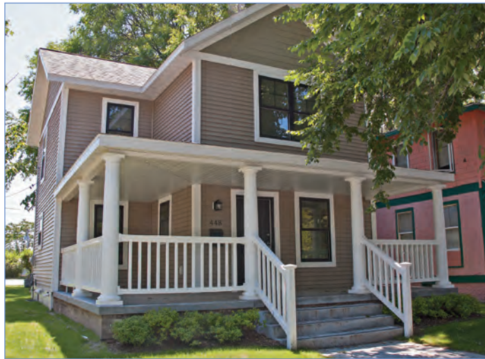
One of 15 units currently being renovated for conversion through the HUD Section 18 - Scattered Sites Program
